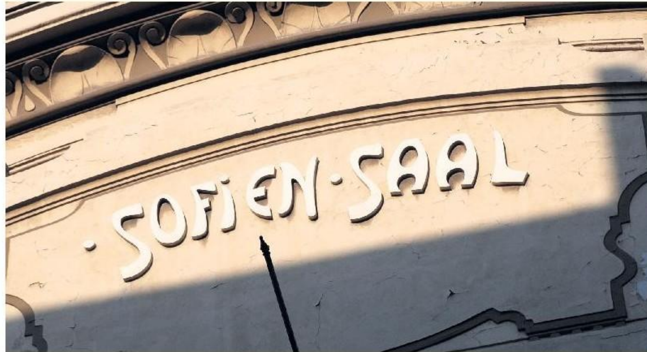
The facade of the Sofiensäle is being refurbished to reflect the original look Photo: Duncan J.D. Smith
